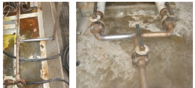
The 2 pictures above show the treated and untreated badly corroded pipeline in Egypt. The treatment was done on 2 km of pipeline.
